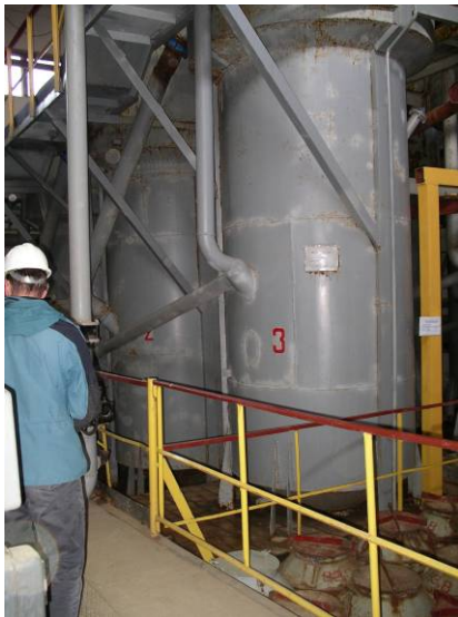
Photo 5. (left) Fluidized bed ion exchange columns
