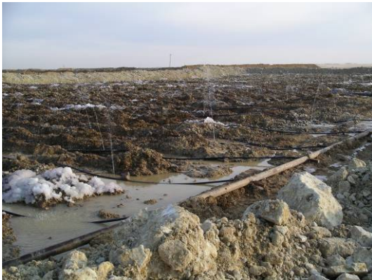
Photo 2 (left). Sprinkling system on the top of the ore heap (white mass on the surface is snow).
